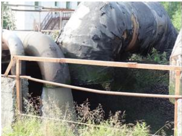
Existing facilities at the Petrozavodsk wastewater treatment plant (photo courtesy of NIB)
