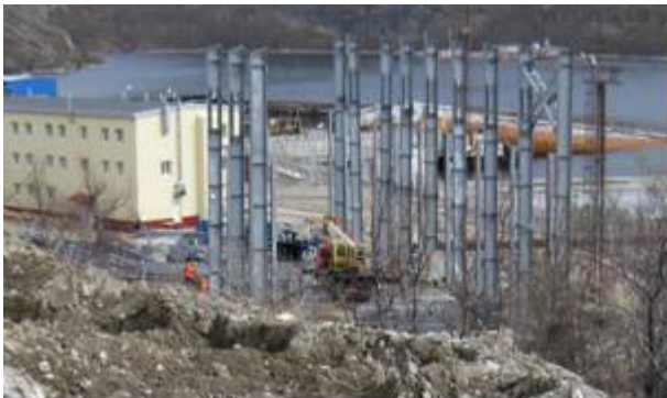
Construction of the Cask Accumulation Pad at Andreeva Bay (Photo courtesy of SevRAO)
