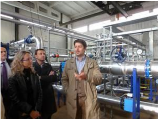
Inside the group heating substation, Mr Pavel Makarov of LLC Shelen describing the refurbishment works.
