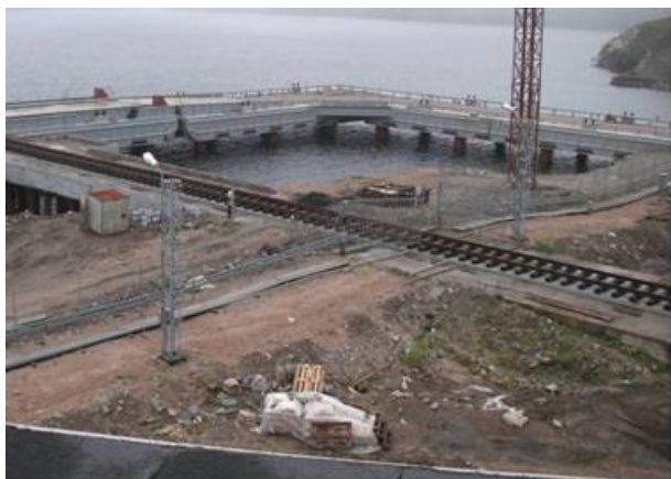
SNF transport infrastructure at the new pier at Andreeva Bay (Photo courtesy of SevRAO)
