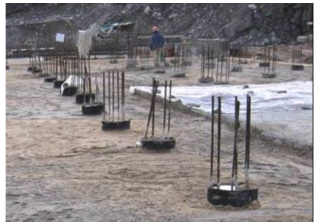
Construction site of the Cask Accumulation Pad at Andreeva Bay (Photo courtesy of SevRAO)
