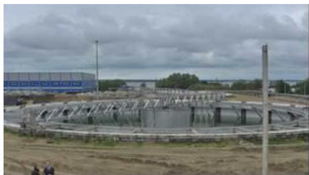
An overview of a new sedimentation tank and a filtration unit on the far left
