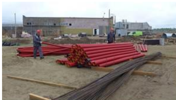
Installation of cable channels. The target is to lay 1800m by end of August 2013.
