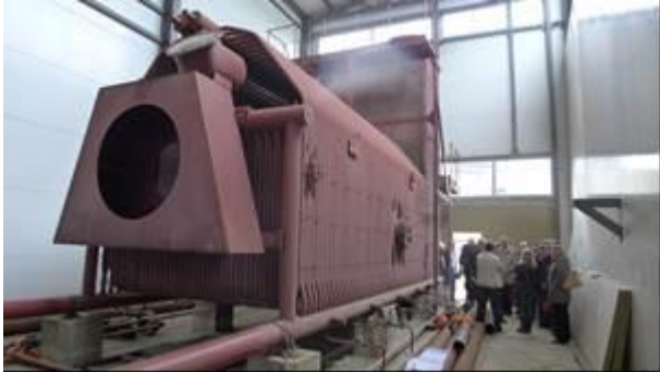
A new gas fired boiler house financed by NDEP grant funds
